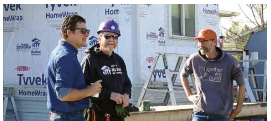
Brad Lancaster (in the hard hat) volunteers on a Helena Area Habitat for Humanity repair job.
